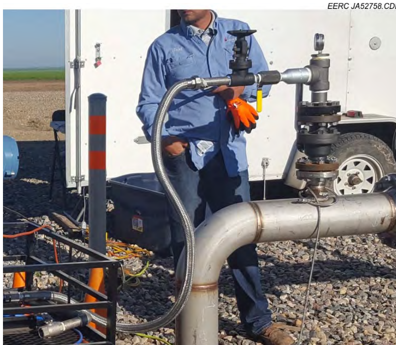
Figure 5. Metering skid connection to the gathering pipeline.
