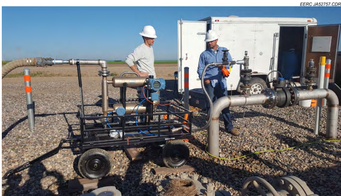
Figure 4. EERC metering skid illustrating connection to a gathering pipeline.
